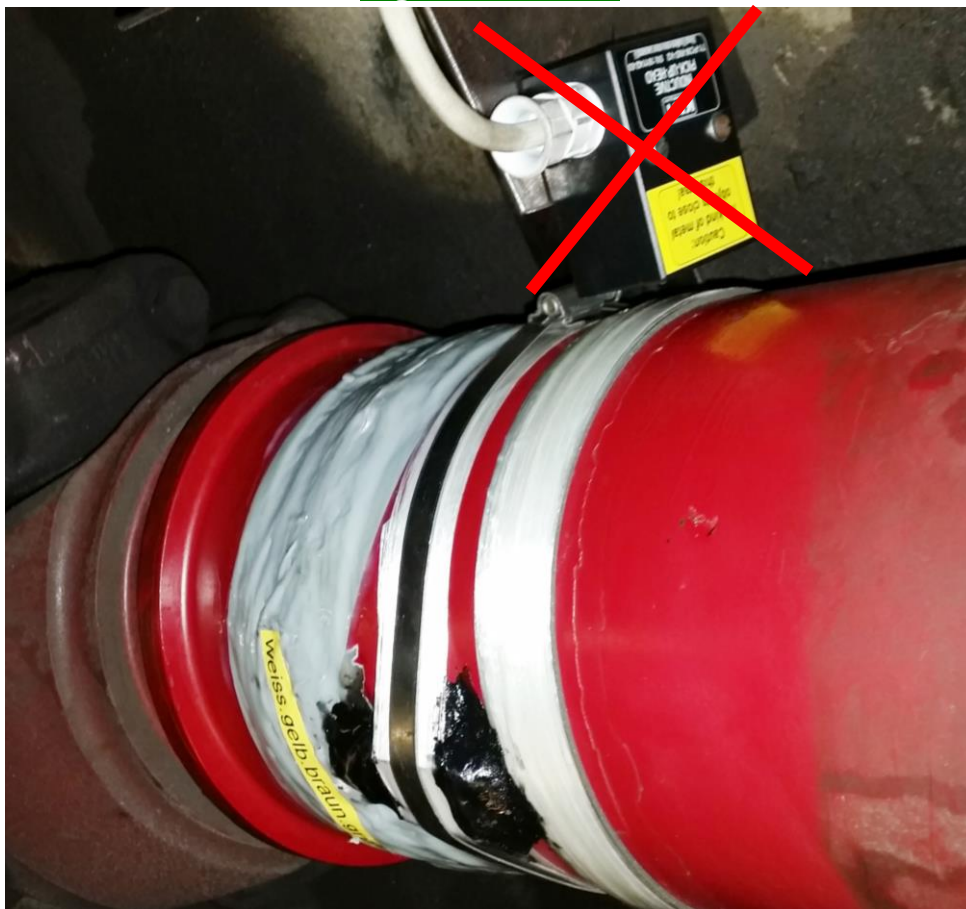
Wrong installation, head position is 90° wrong to the coil and will not work!
